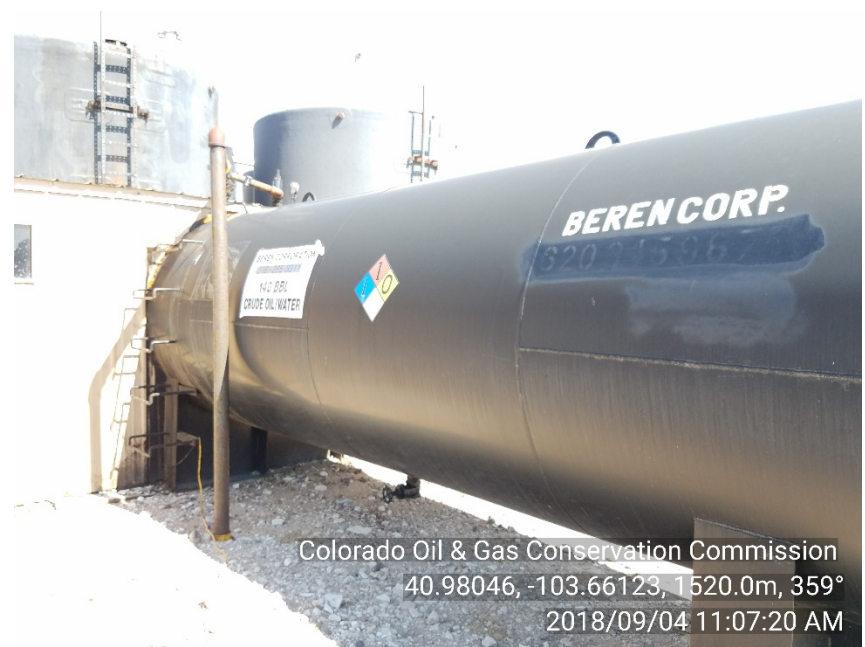
Photo #4 Moyer Unit Battery Free Water Knockout
