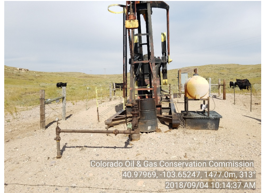
Photo #2 Moyer Unit 16-29 wellhead Stained soil appears to be remediated Bradenhead needs plumbed to surface
