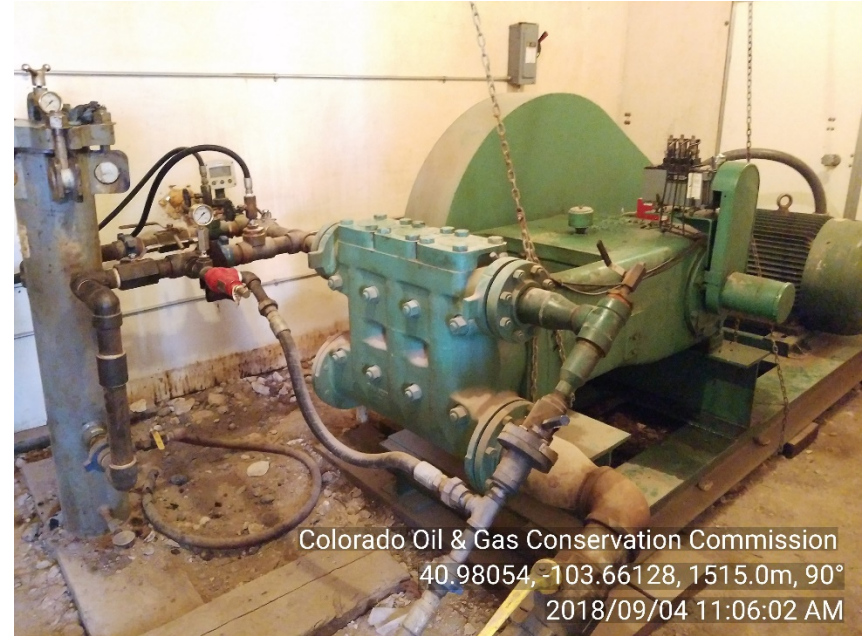
Photo #9 Moyer Unit Injection Facility Injection pump
