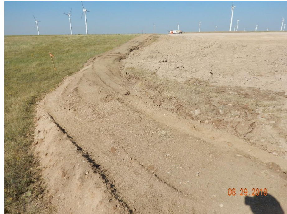
Photo 12: Photo taken from southeast end of the location, facing west. Photo shows the stormwater ditch along the perimeter of the location.
