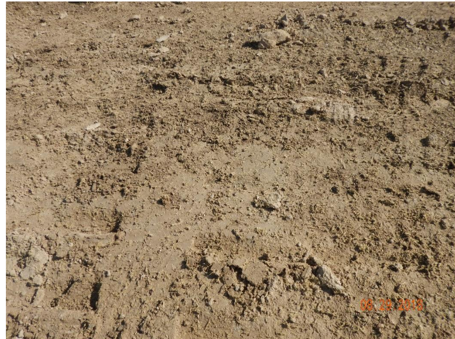
Photo 6: Continued from photo 5. Photo shows ditch/berm has been properly compacted. Additionally, operator has applied a Tackifier for additional soil stabilization.
