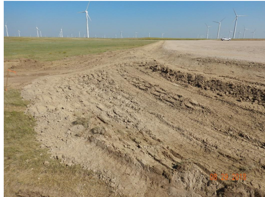
Photo 20: Photo taken from the southwest corner of the pad, facing north. Photo shows the stormwater ditch along the western perimeter of the pad
