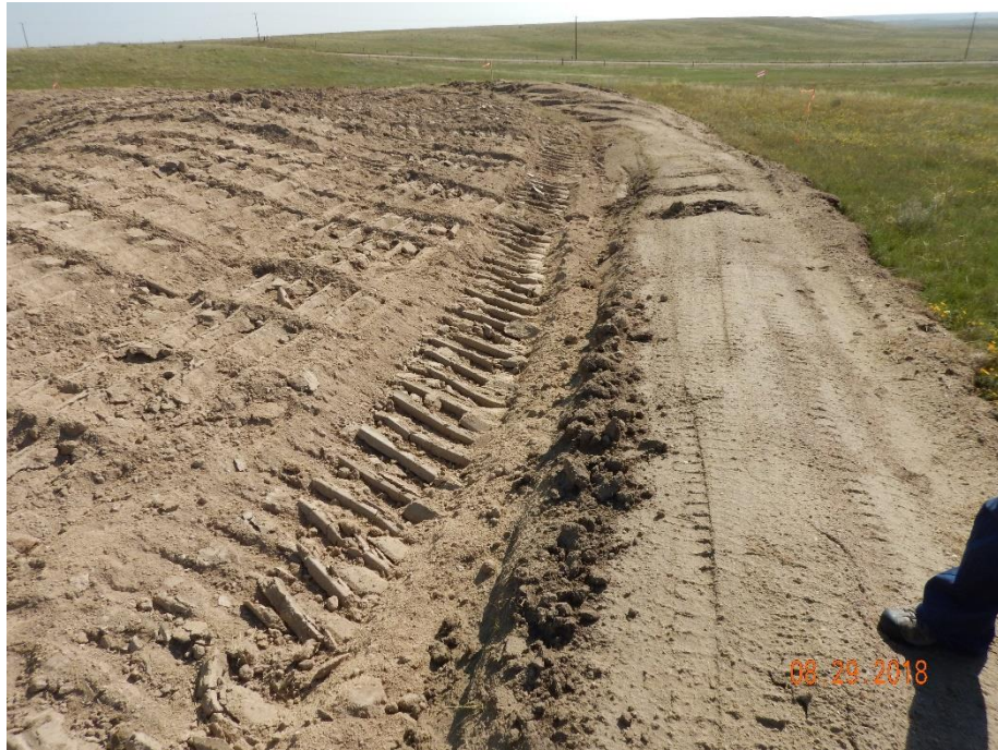
Photo 13: Photo taken from the southeast end of the location, facing east. Photo shows a portion of the sediment pond/trap on the southeast corner of the pad. BMP does appear to have been installed in conjunction with the perimeter ditch as a secondary control, however, it is noted that pond does not appear to have sufficient inlet protection, or a protected outlet to allow for sediment laden-free stormwater discharge from the location in accordance with good engineering practices.
