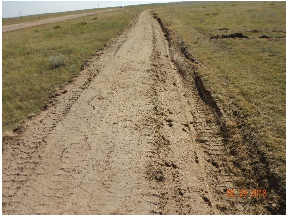
Photo 5: Photo taken from the north end of the location, facing east. Photo shows the stormwater control ditch and berm operator has installed along the perimeter of the location.
