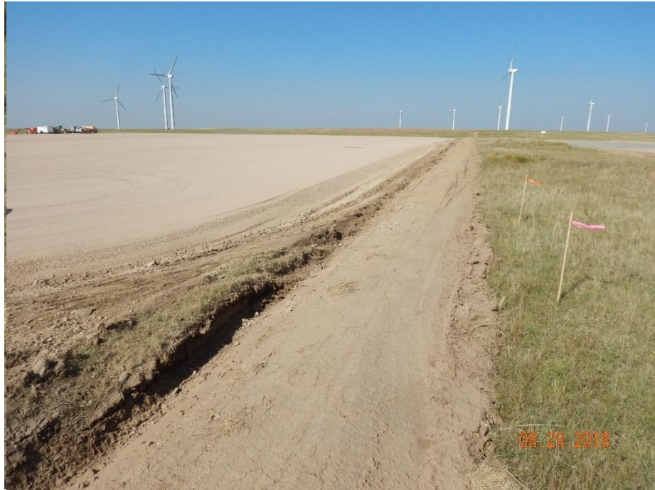
Photo 1: Photo taken from the north end of the location, facing west. Photos 1-5 provide an overview of the construction site from west, to southwest, to southeast, to east.
