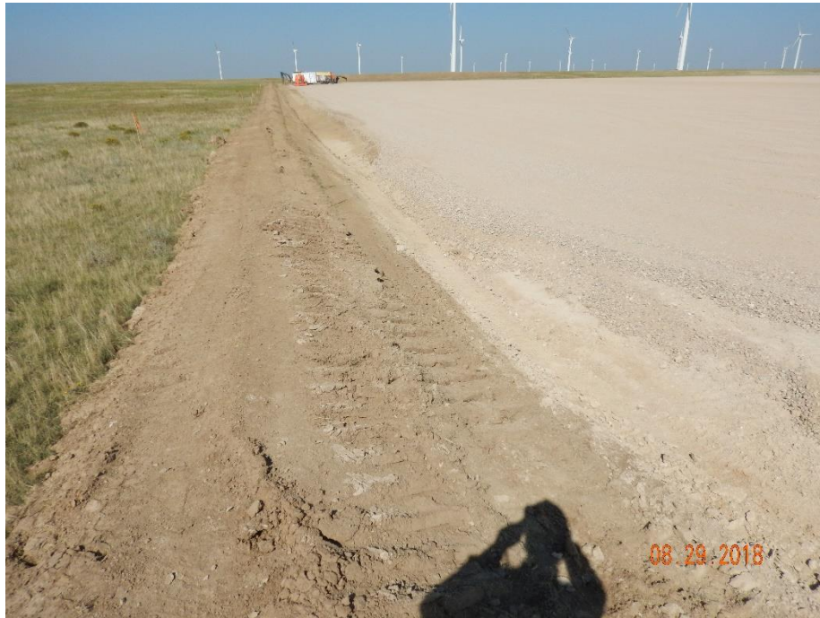
Photo 17: Photo taken from the southeast corner of the pad, facing east. Photo shows perimeter stormwater control ditch along the perimeter of the pad. Ditch appears to have been properly constructed and compacted. Operator also implemented a Tackifier on ditch/berm for additional stabilization.
