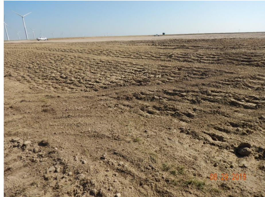
Photo 22: Photo taken from the west end of the pad, facing northeast. Photo shows slopes have been tracked and a tackifier applied for stabilization.
