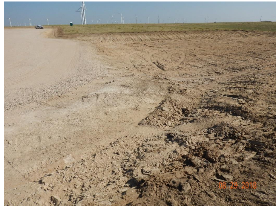
Photo 18: Photo taken from southwest corner of the sediment trap/pond. Photo shows BMP does not appear to have inlet protection in accordance with good engineering practices. See comments under photo 13.
