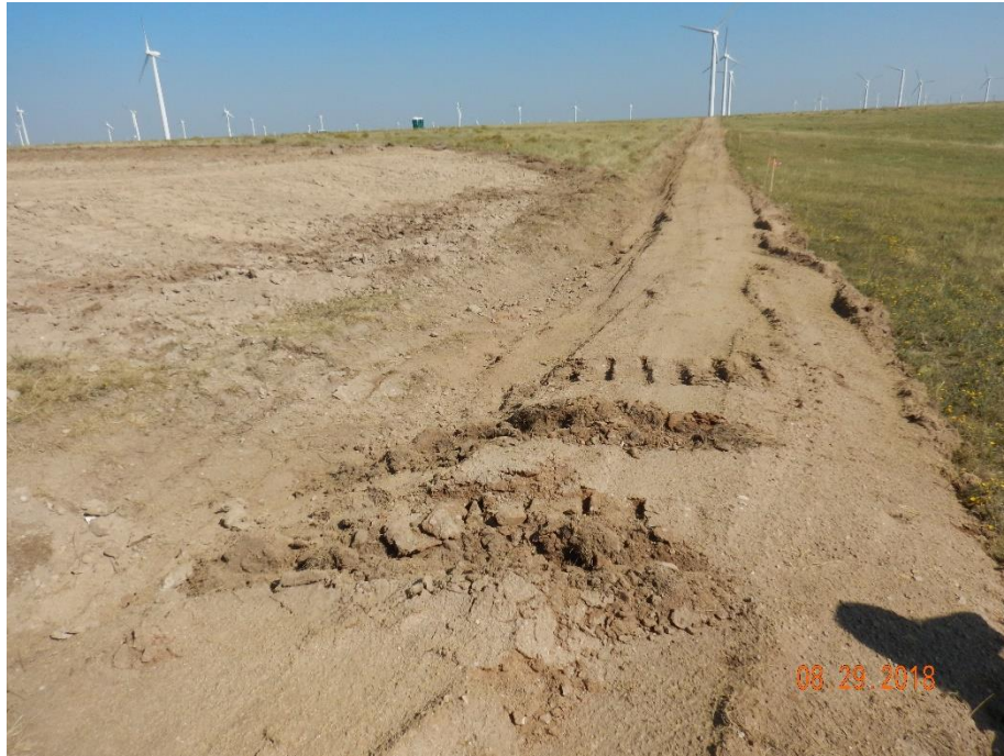
Photo 11: Photo taken from southeast end of the location, facing north. Photo shows the stormwater ditch along the perimeter of the location. Photo also shows that ditch/berm appear to have been traveled over compromising the integrity of the BMP. Advise maintenance. It is also noted that this area of the ditch appears to be the lowest point of the location. The perimeter control does not appear to have an outlet-area to allow for sediment laden-free stormwater discharge from the location.
