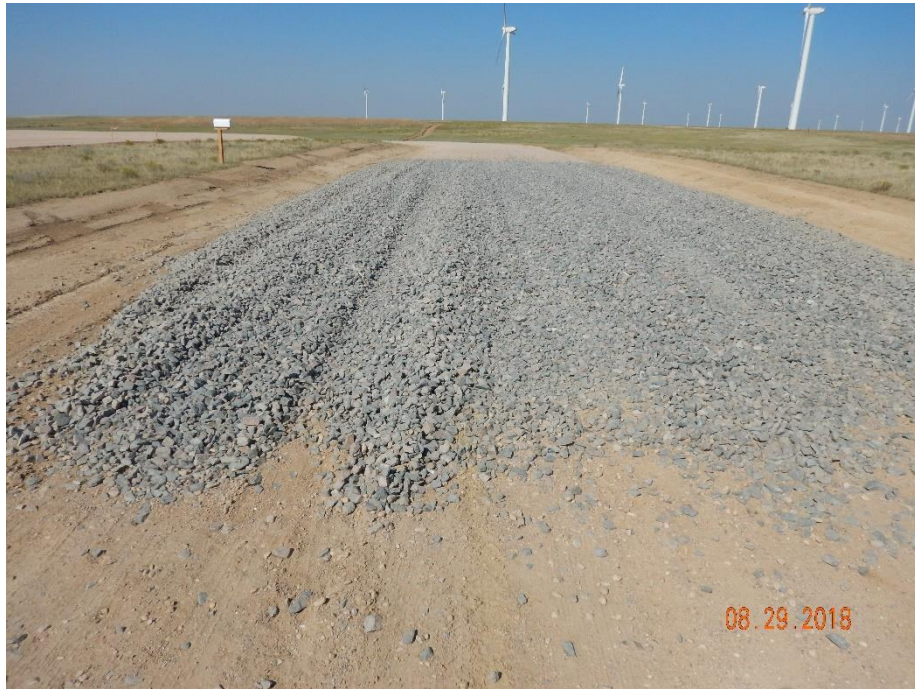
Photo 27: Photo taken from the access road, facing west. Photo shows tracking pad.
