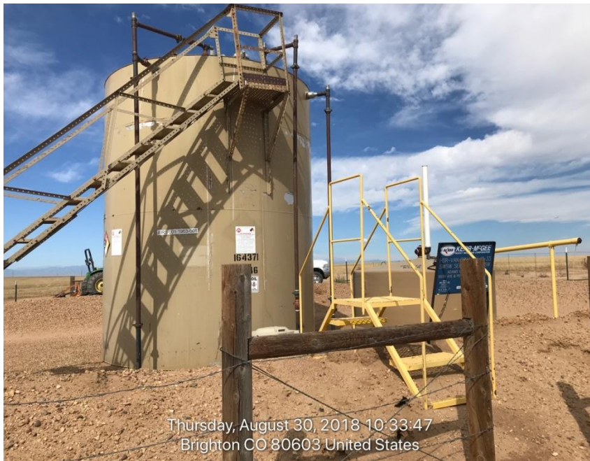
Photo#1 Production Tank and Produced Water Pit
