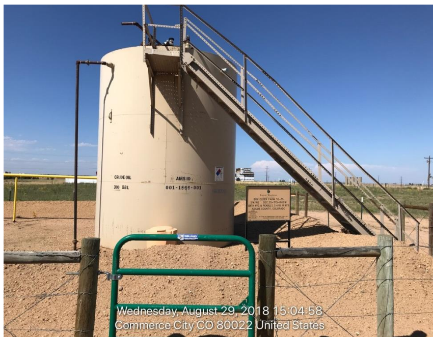
Photo#1 Production Tank
