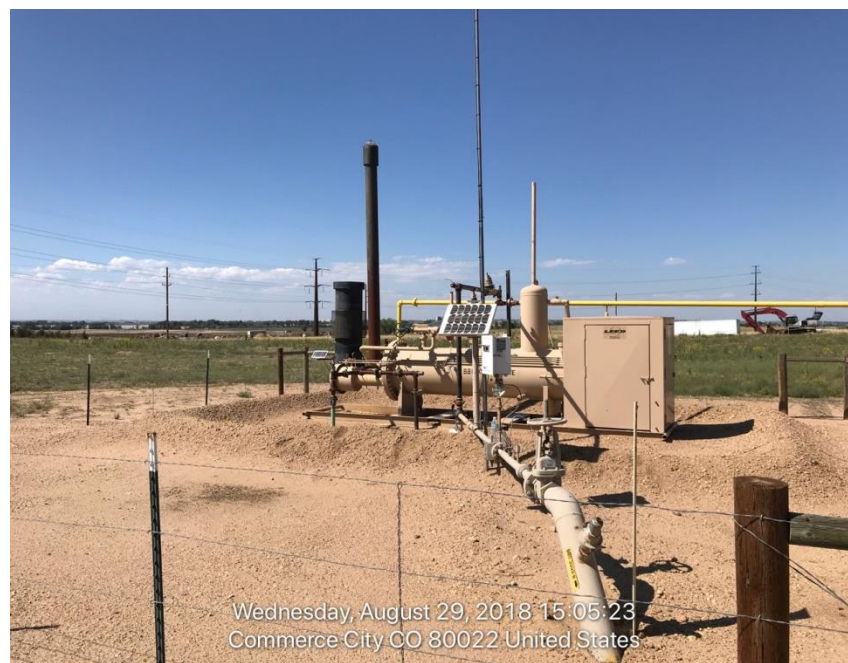
Photo#2 Separator/Gas Meter/ECD
