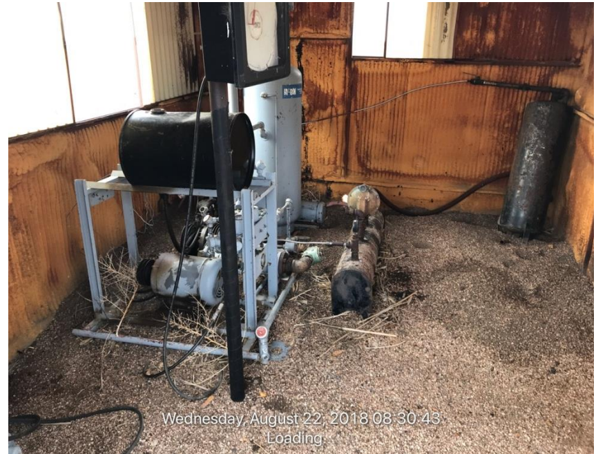
Photo#2 Corrective Action/Unused Equipment
