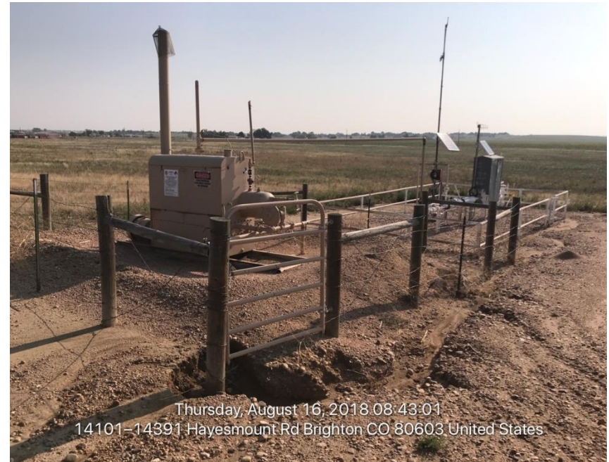
Photo#2 Separator and Gas Meter
