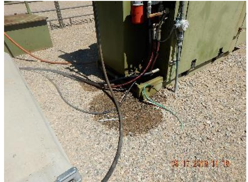
Photo 2: Impacted soil and gravel at front of OilLift unit.
