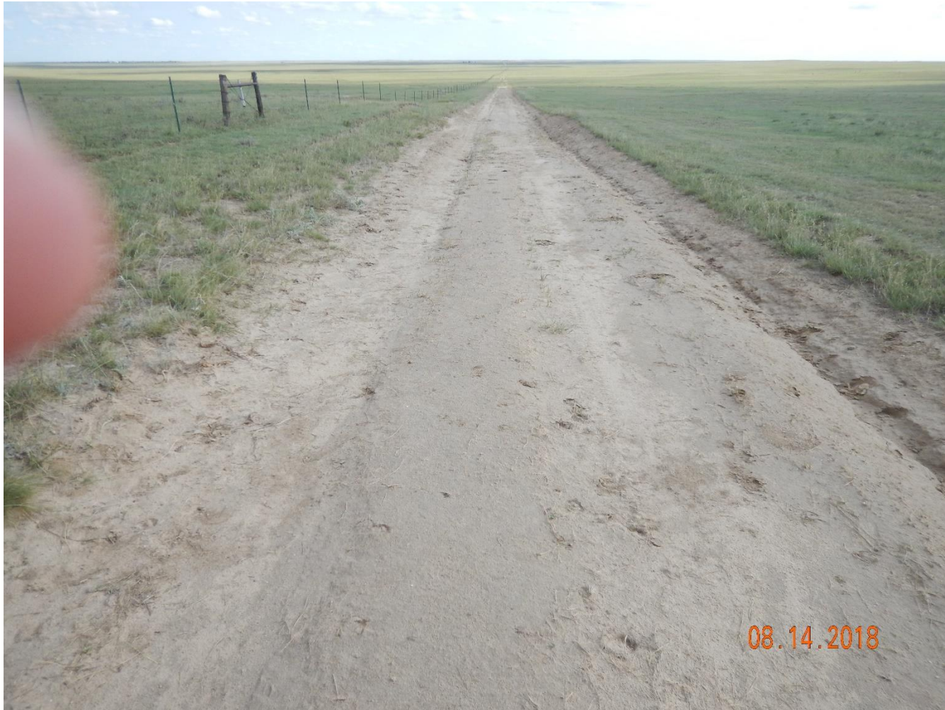
Photo 1: Photo taken from the access road, northeast of the location, facing south. Previous inspection documented erosion degradation concerns on access road. Photo shows maintenance has occurred on access road.
