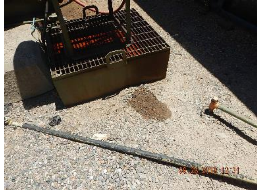
Photo 8: Impacted soil and gravel at lube oil tank previous inspection.
