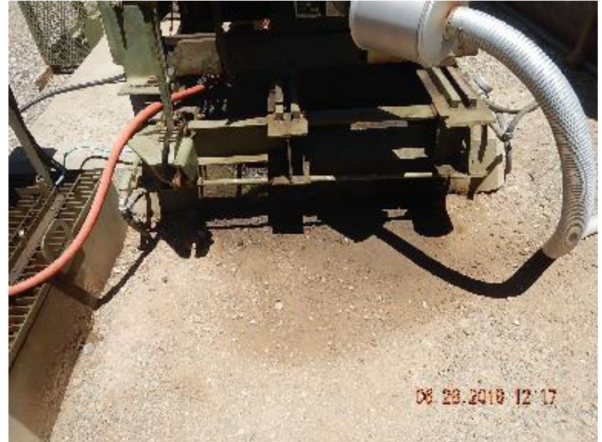
Photo 4: Impacted soil and gravel at rear of pump jack from previous inspection.
