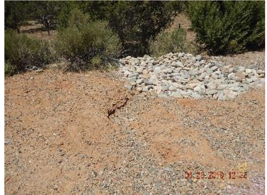
Photo 10: Erosion channel at front of rock run down from previous inspection.
