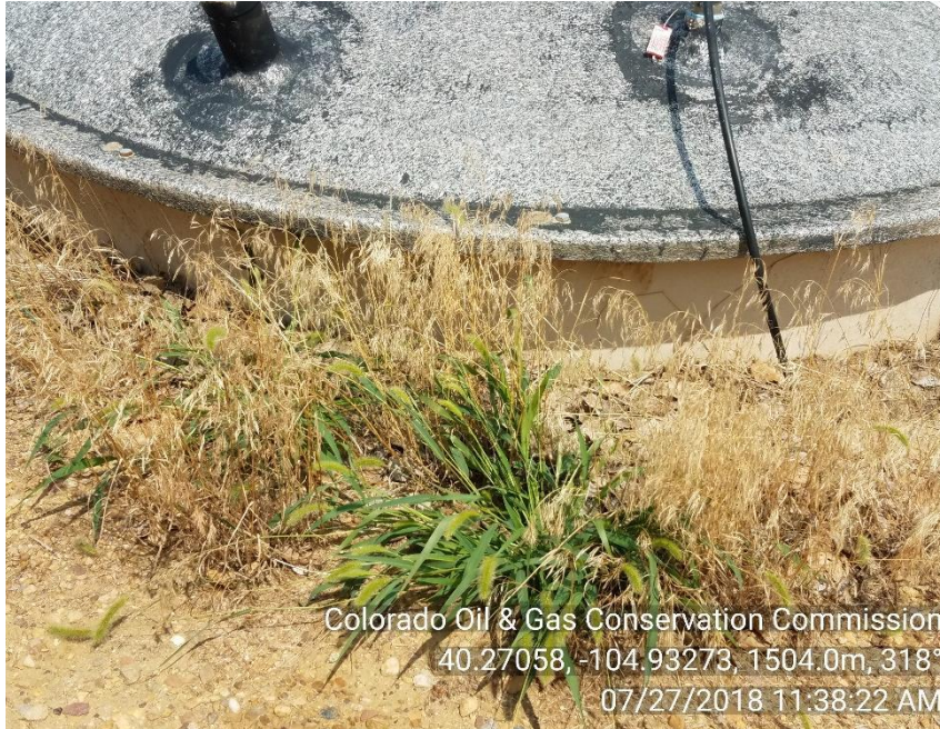
Weeds by tank before completed CA
