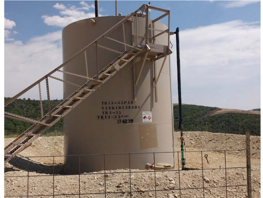
Condensate tank in dirt SPCC looking SE
