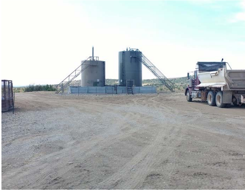
New tank battery looking south
