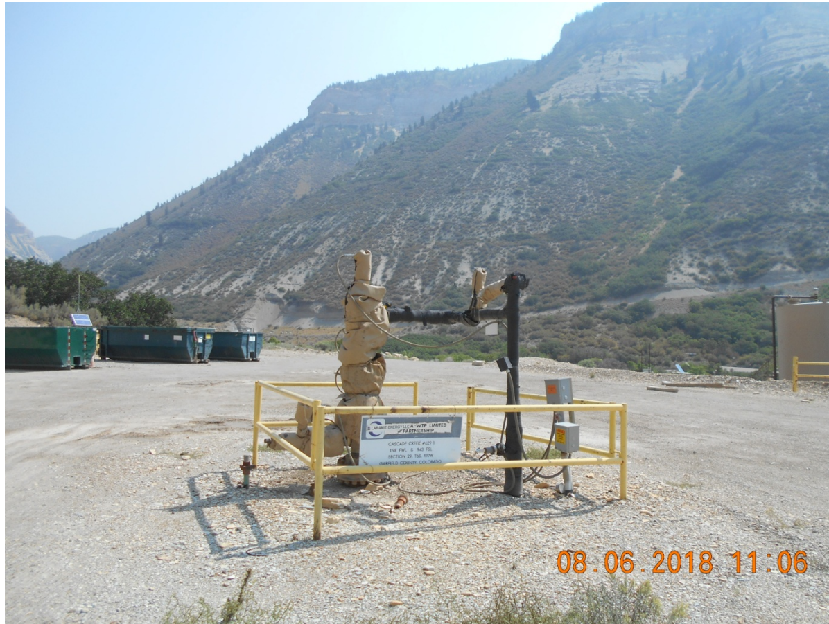
Injection wellhead with sign
