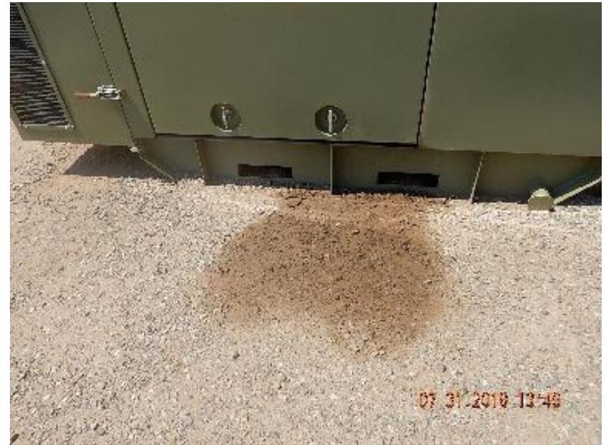
Photo 2: Impacted soil and gravel at OilLift generator.
