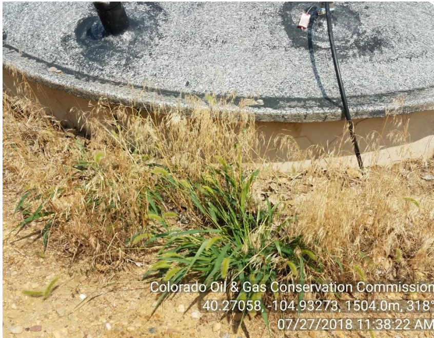
Weeds around produced water tank.
