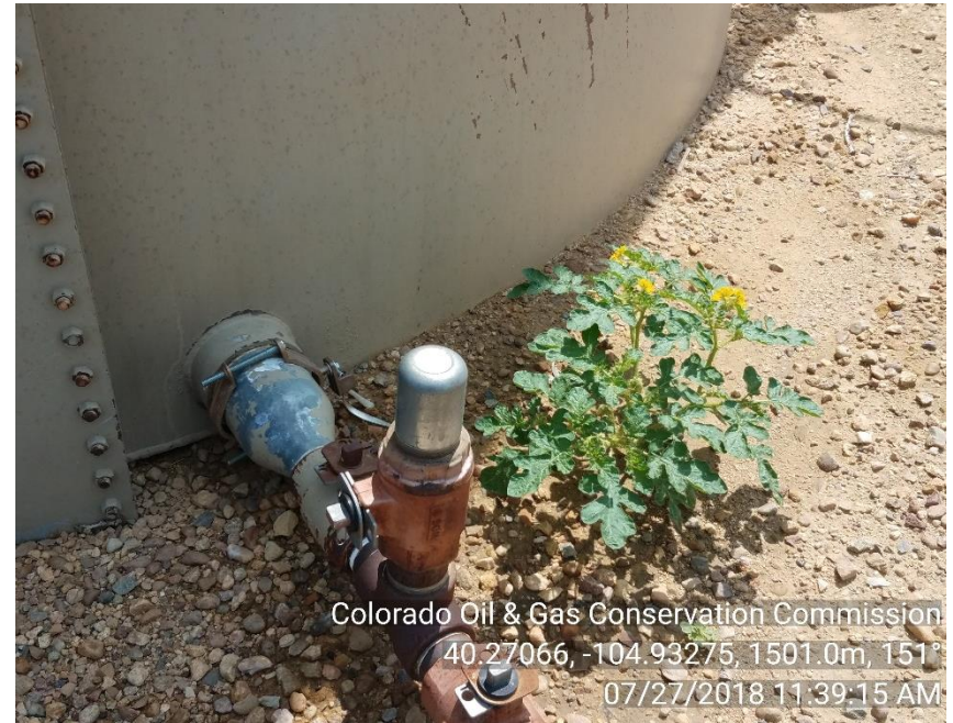
Weeds around crude oil tank
