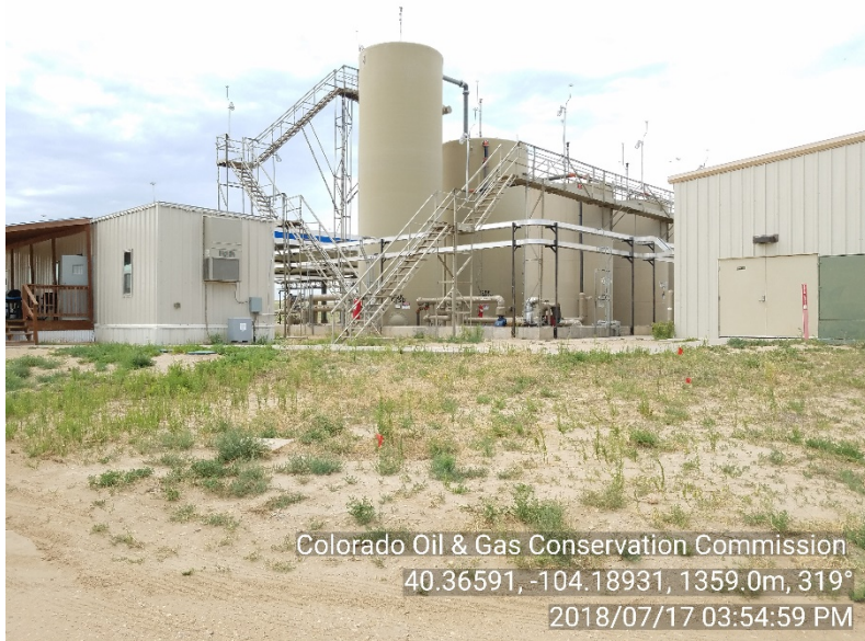
Photo # 7 NGL C11 (API 05-123-38533) Injection Facility View 2
