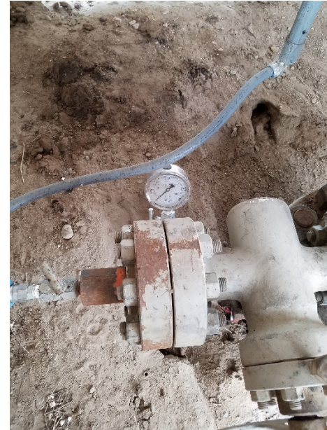
Photo #4 NGL C11 (API 05-123-38533) injection wellhead Bradenhead psi: 0#
