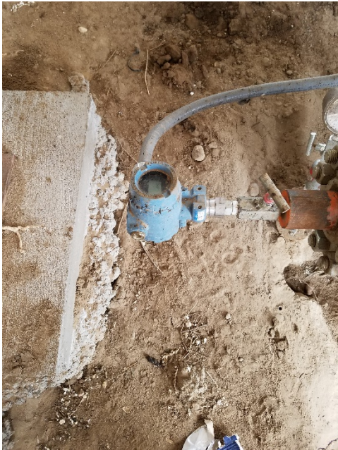
Photo #3 NGL C11 (API 05-123-38533) injection wellhead Casing Press: 0#
