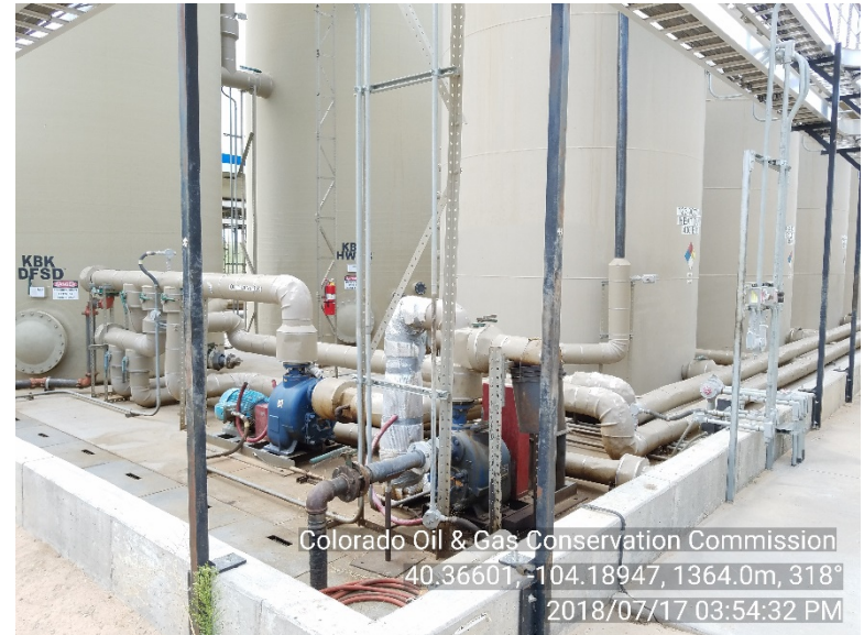
Photo #8 NGL C11 (API 05-123-38533) Tank area
