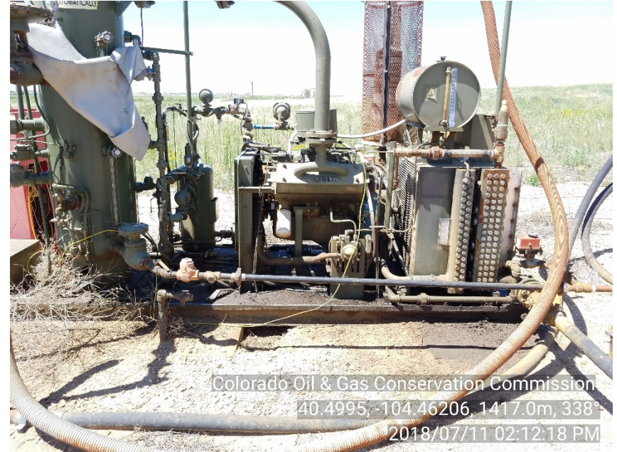
Photo #4 Compressor Stained soil
