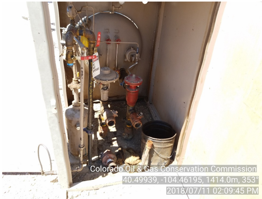
Photo #3 East separator doghouse. Trash
