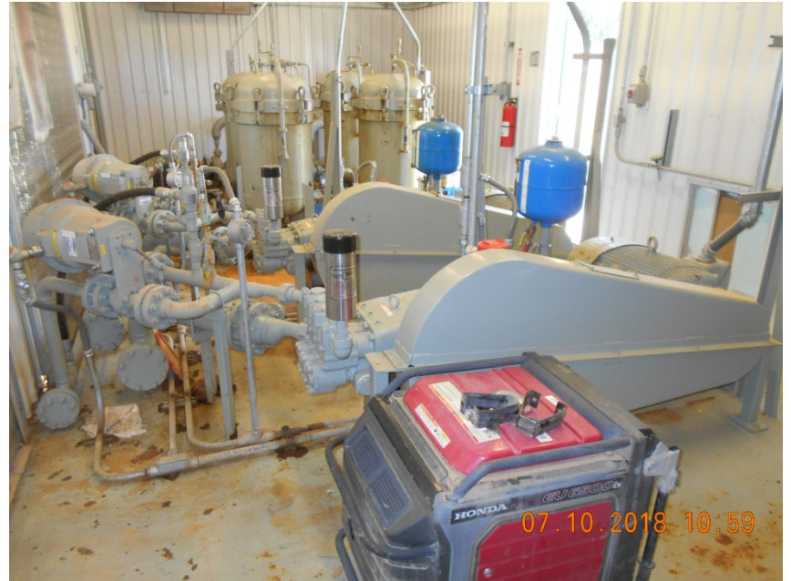
Pumps inside housing
