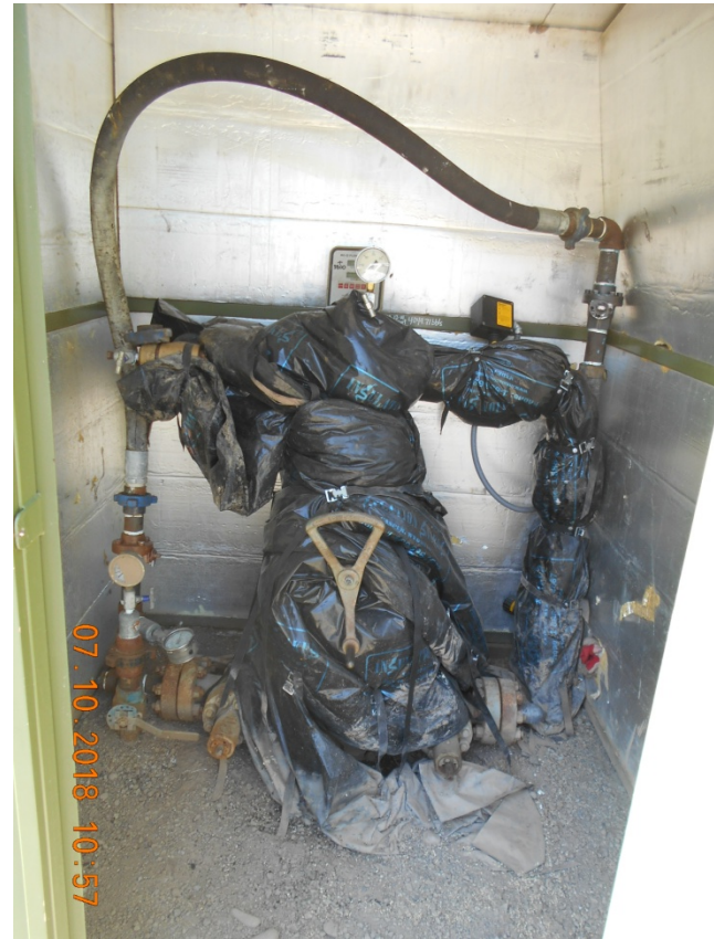
Wellhead inside housing
