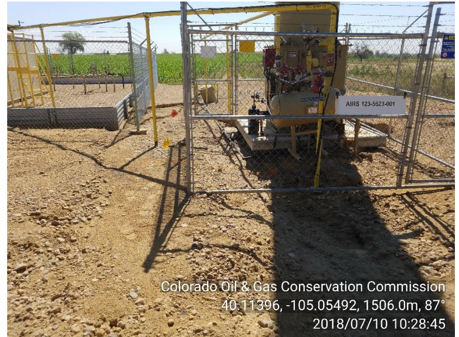
Photo 4. Erosion undermining emission control device platform
