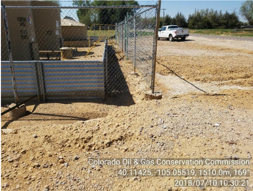
Photo 5. Erosion under tank battery containment
