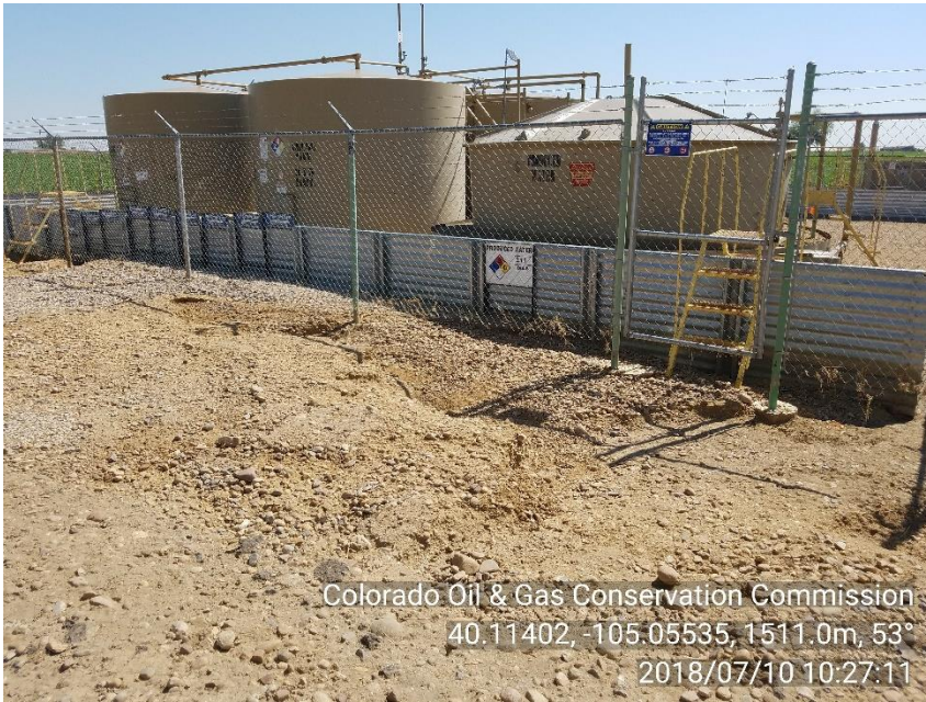
Photo 3. Erosion under tank battery containment
