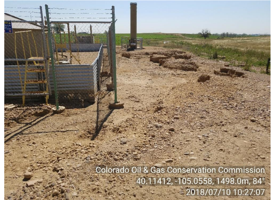
Photo 2. Erosion south side of battery
