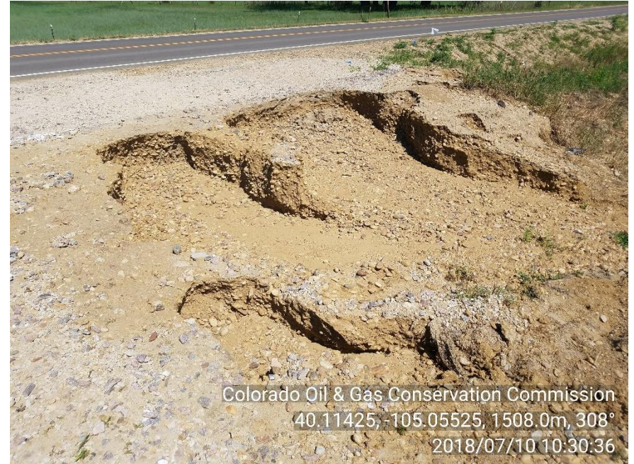
Photo 4. Erosion on entrance to tank battery
