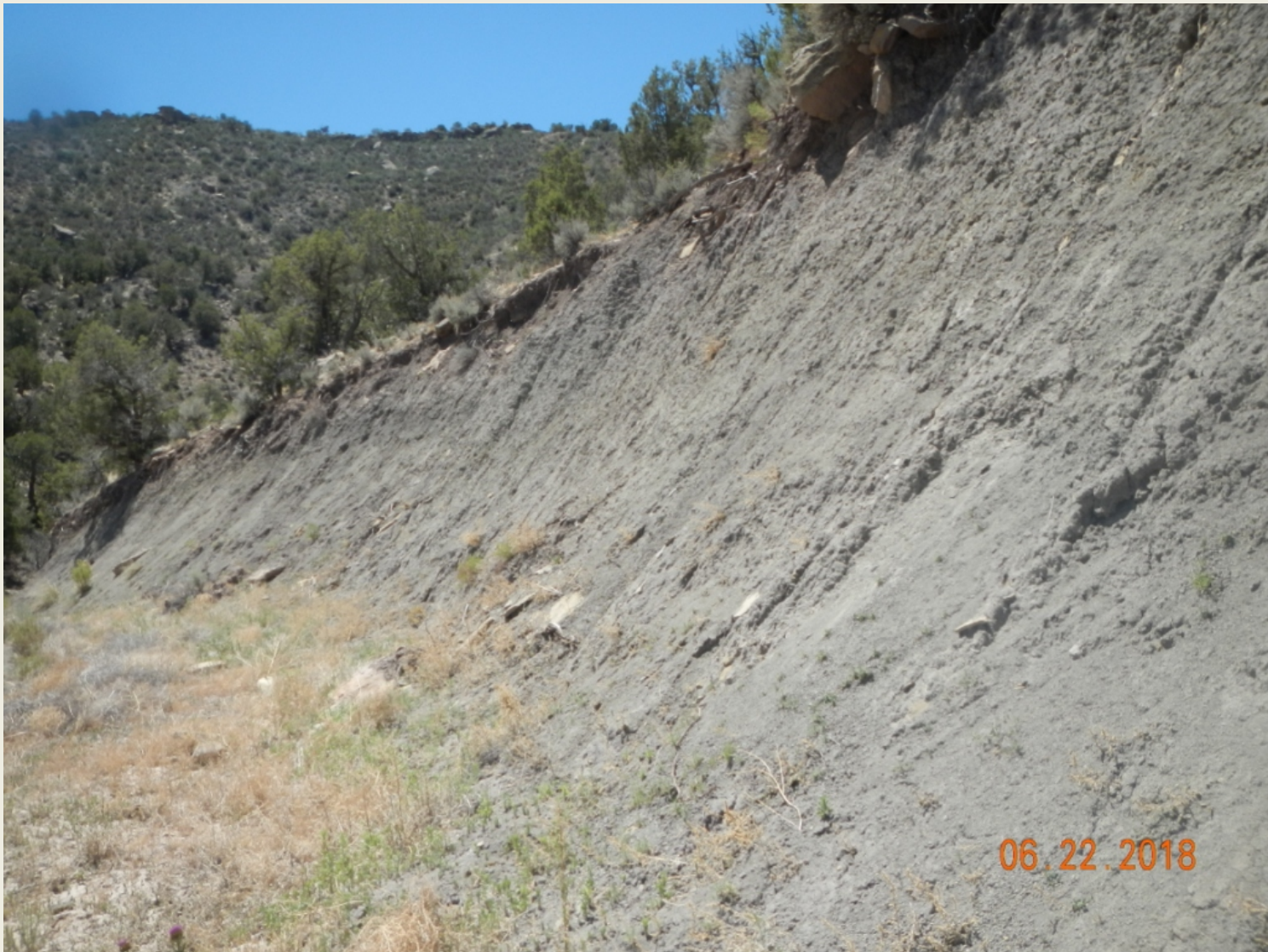
Photo 3. View of cut-slope approximately 20 feet tall along the western edge of the project area. Proper recontouring and revegetation is needed to stabilize this slope. Vegetation undercutting at the top of the slope, and sediment deposition at the toe of the slope are evidence that the slope is actively eroding.
