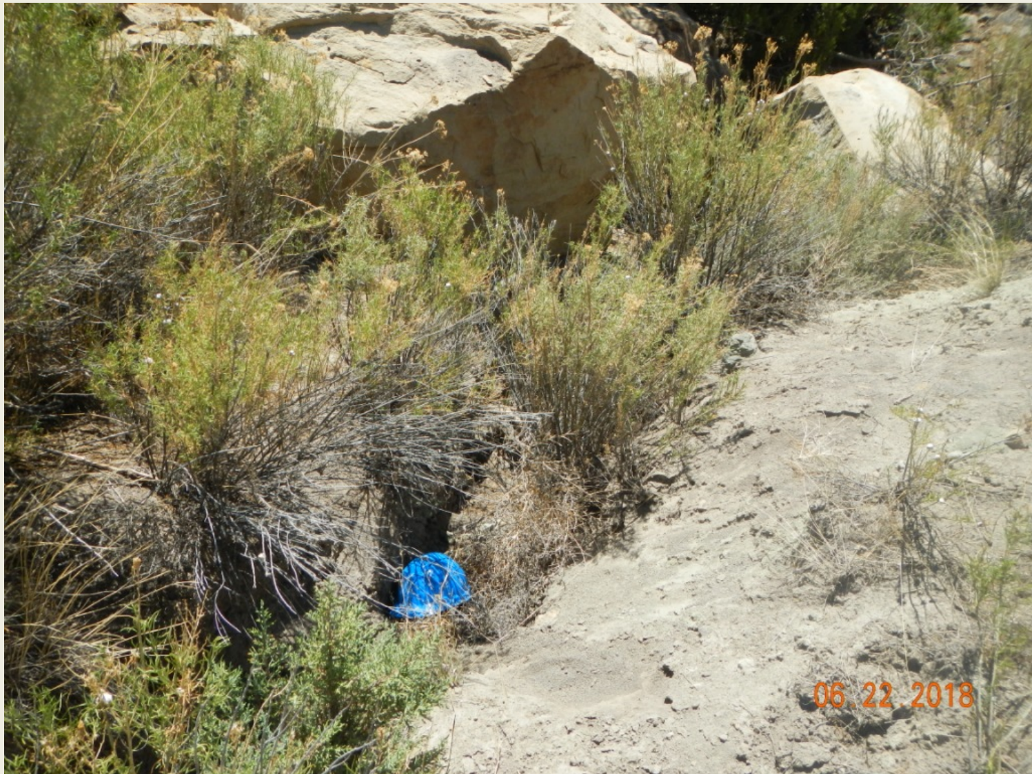
Photo 7. View of erosional channel approximately 2.5 feet deep and 2 feet deep along the southern edge of the project area.
