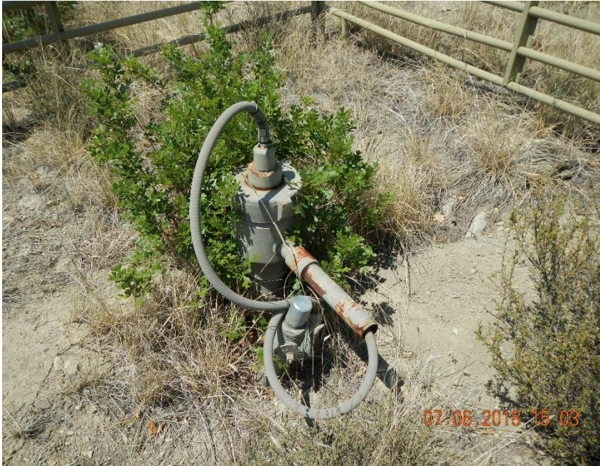
Highway 151 34-4-30 #1 well head.
