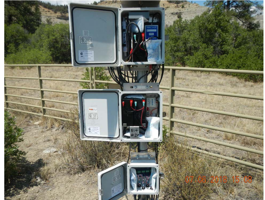
Equipment enclosures with desiccants replaced.
