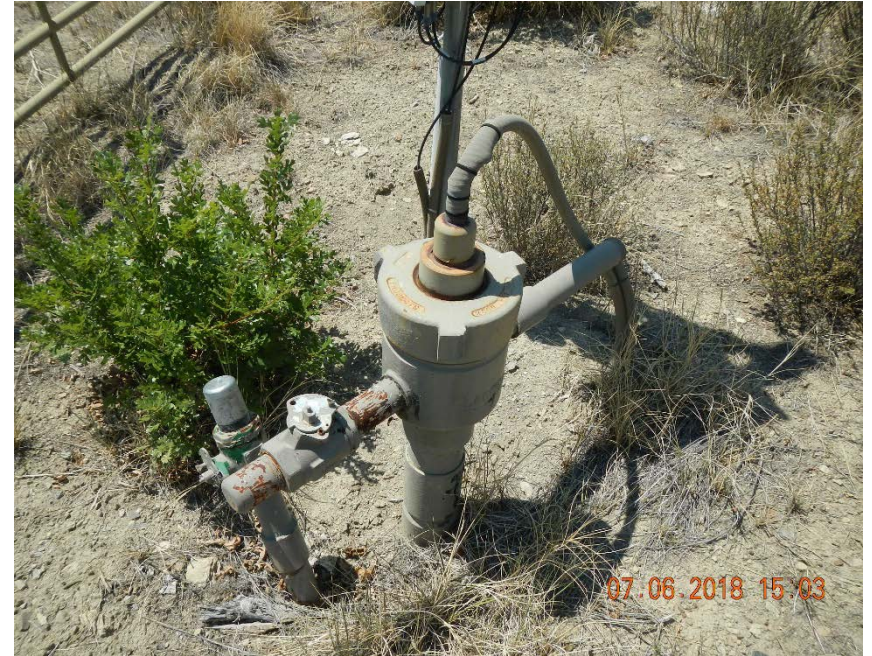
Highway 151 34-4-30 #2 well head.
