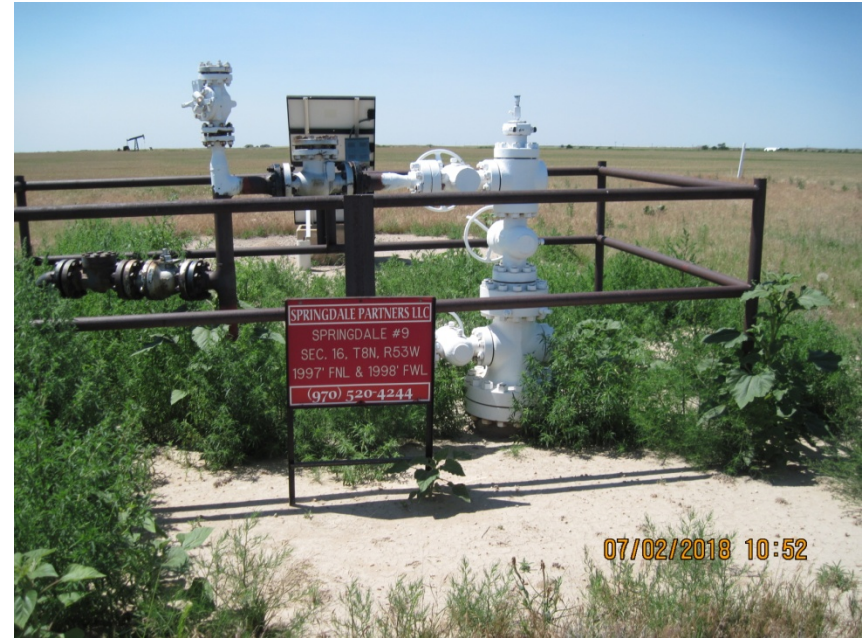
2. Wellhead & solar panel
