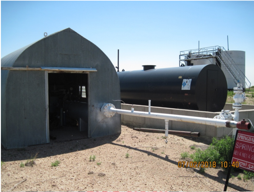
3. Horizontal heater treater & Free water knockout
