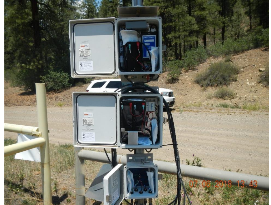
Equipment enclosures with desiccants replaced.
