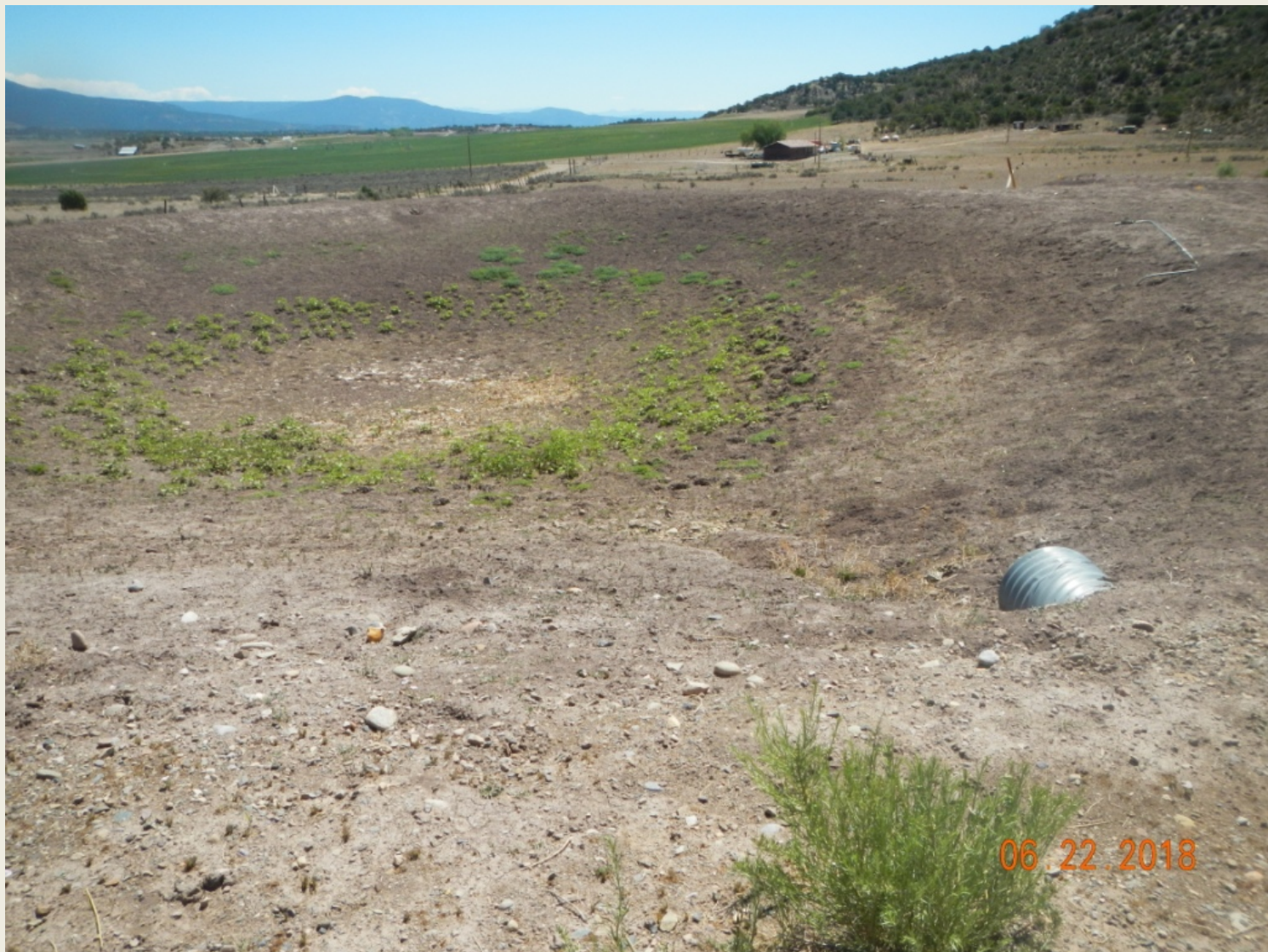
Photo 7. View of silt trap in the northeastern portion of the project area.
