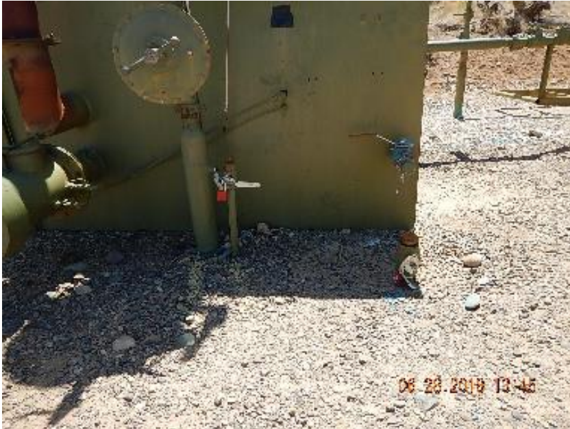
Photo 3: Unused risers at separator.
