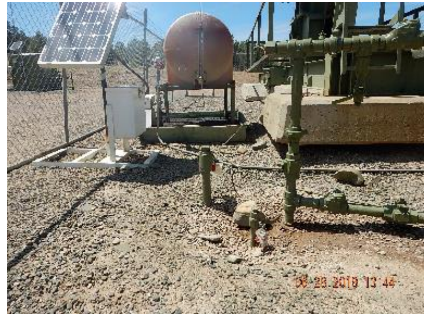
Photo 2: Unused risers at wellhead.
