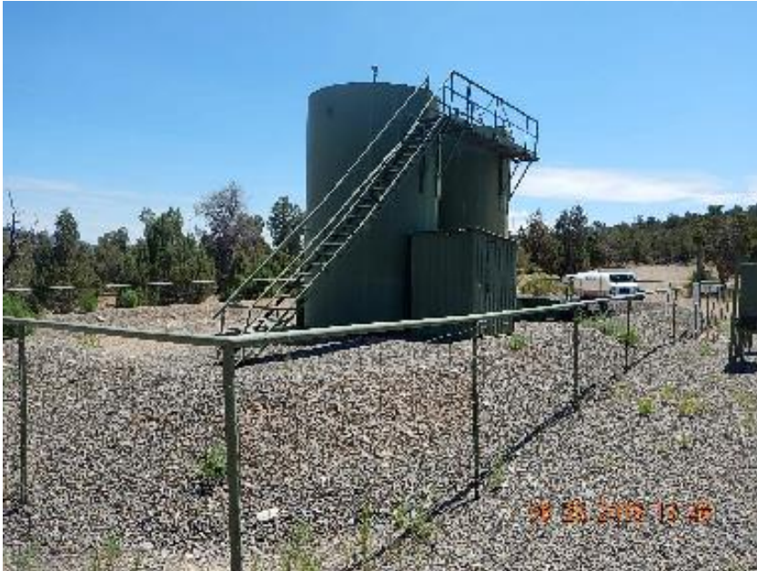
Photo 5: Tank battery overview.
