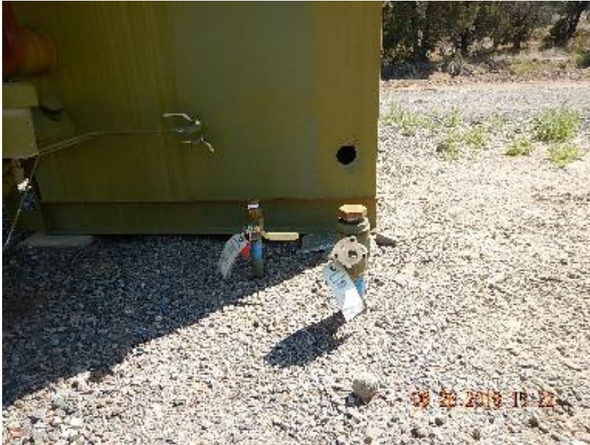
Photo 3: Unused 1" (B) point and unused 2" (B) point steel risers at #5-5 separator.
