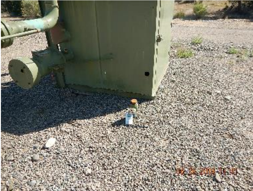
Photo 7: Unused 3" steel riser (B) point at #8-2 separator.
