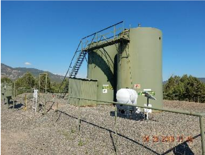
Photo 9: Tank battery overview.
