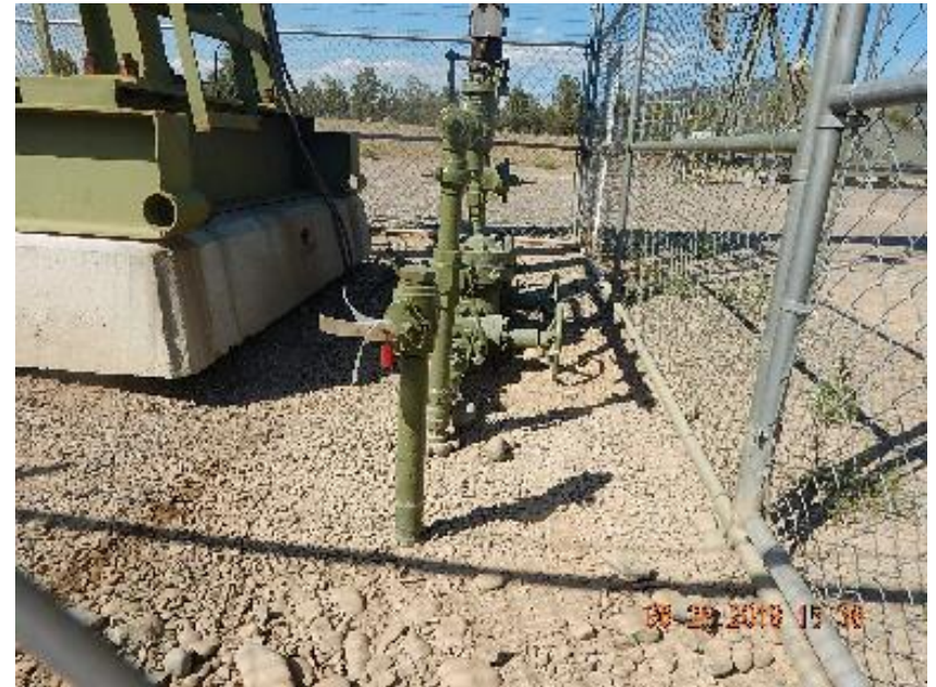
Photo 6: Unused 3" steel riser (A) point at #8-2 wellhead.
