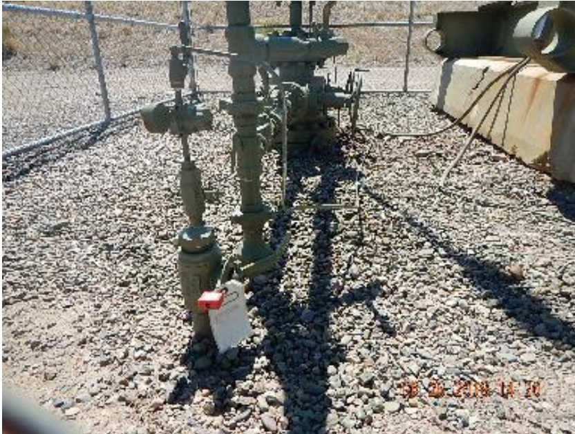
Photo 5: Unused 3" steel riser at #8-3 wellhead.
