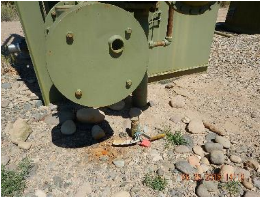
Photo 3: Unused 1" steel supply gas riser (A) point at #5-1 separator.
