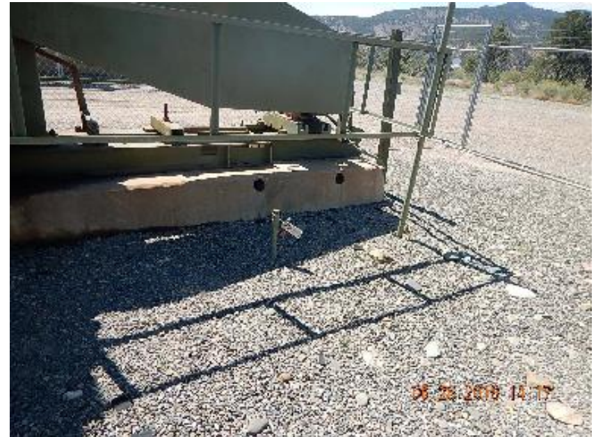
Photo 2: Unused 1" steel supply gas riser (B) point at #5-1 wellhead.
