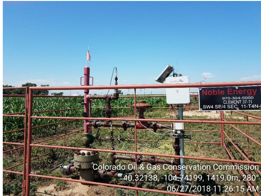
Photo of wellhead
