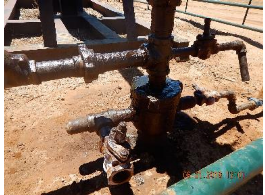
Photo 4: Impacted soil at wellhead.
