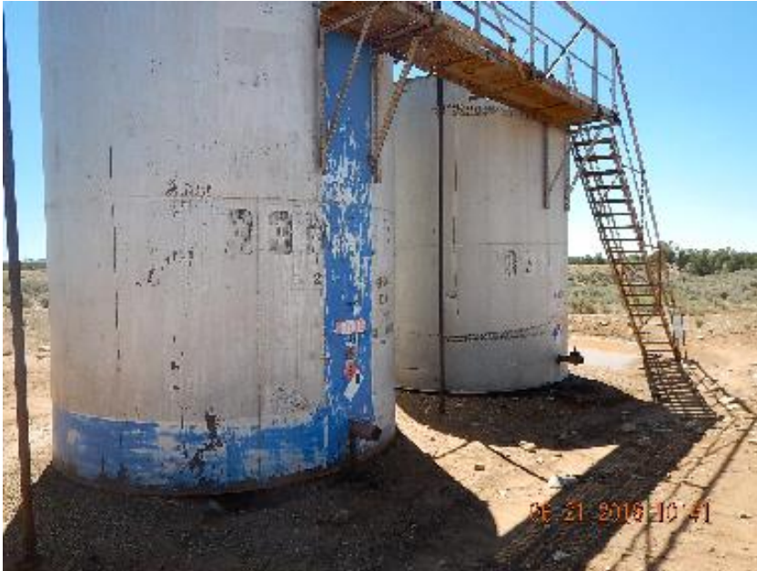
Photo 3: Tank battery overview.
