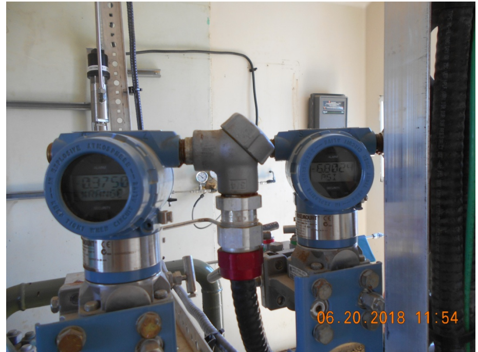
Injection wellhead tubing gauge
