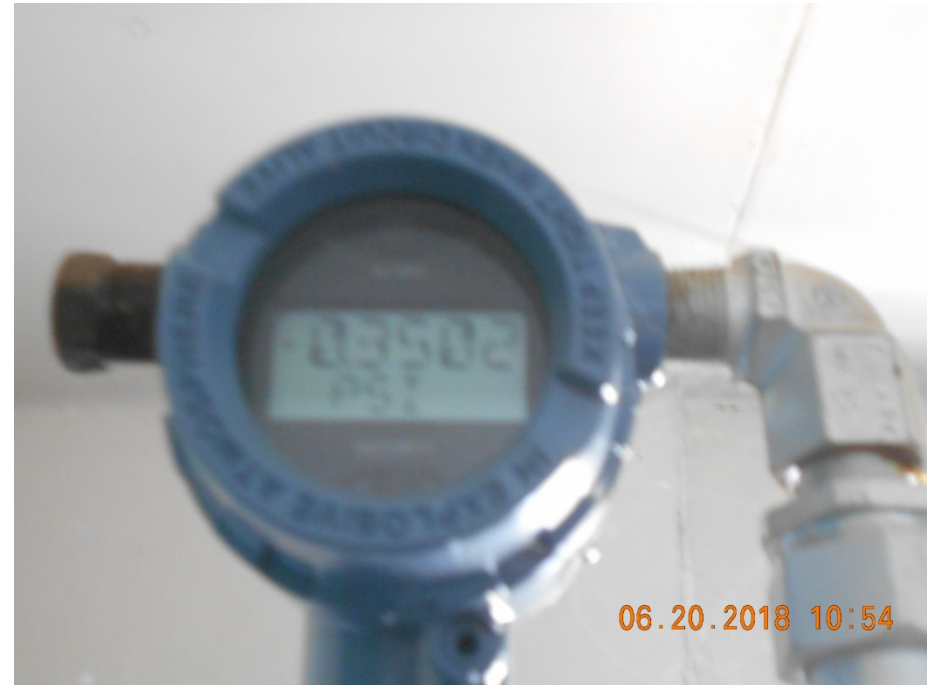
Injection wellhead tubing gauge
