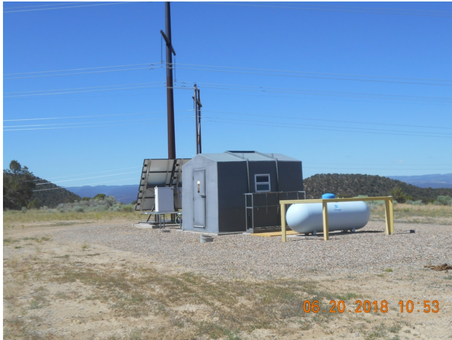
Injection wellhead housing
