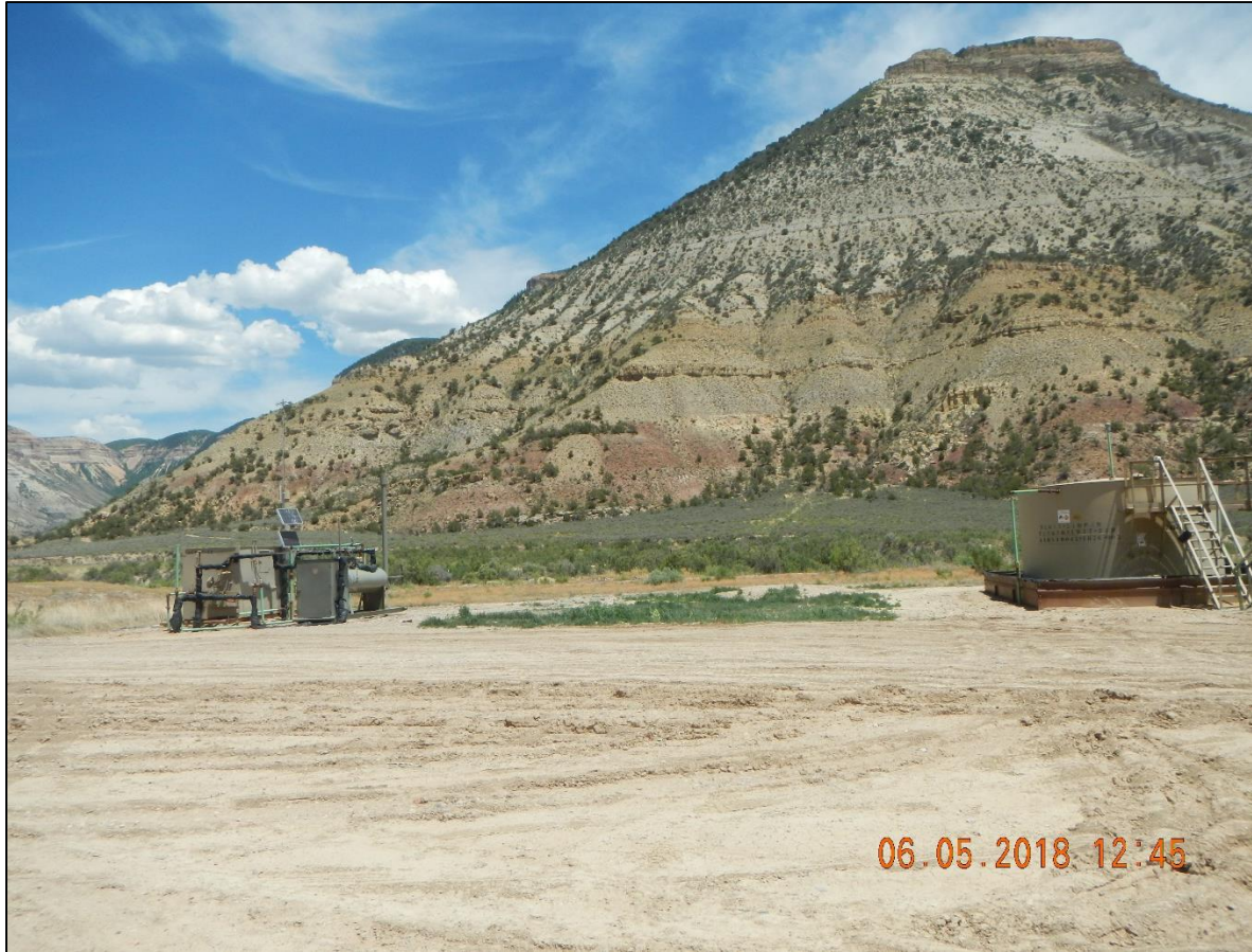
Separator and tanks.
