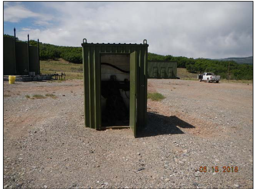
Photo 2. Wellhead in shelter.
