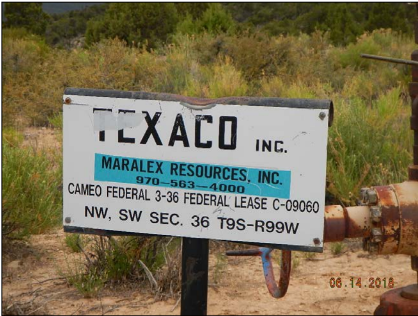
Photo 1. Wellhead sign is missing public road used to access the site.
