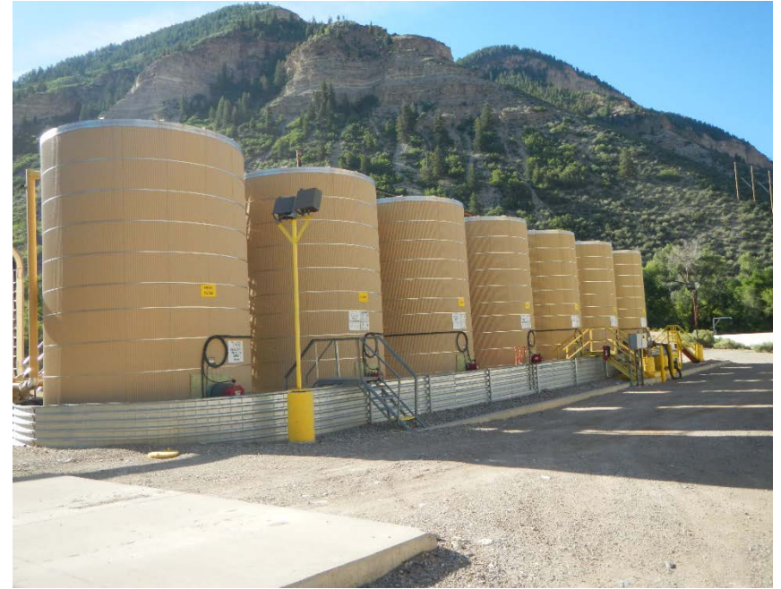
Condensate ASTs looking southeast
