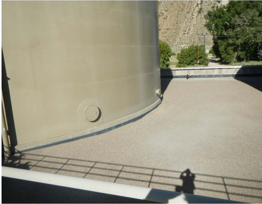
80K bbl AST within secondary looking west
