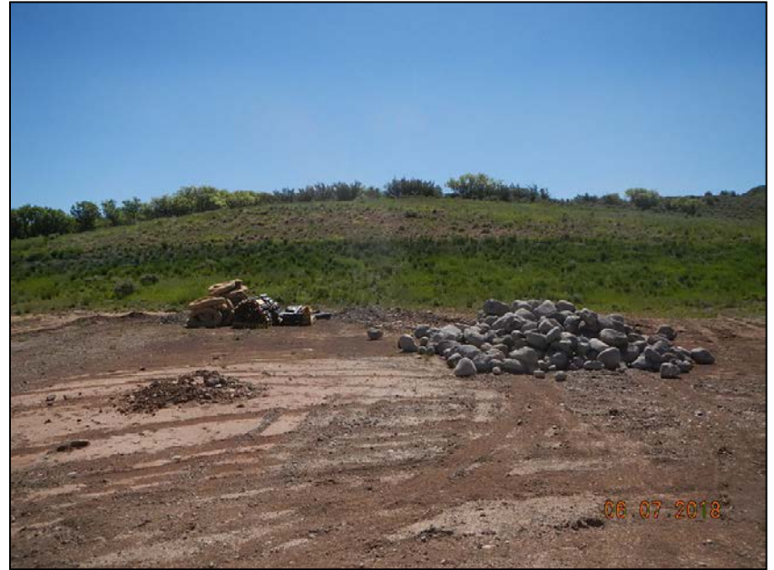
Photo 2. Stored stormwater materials.
