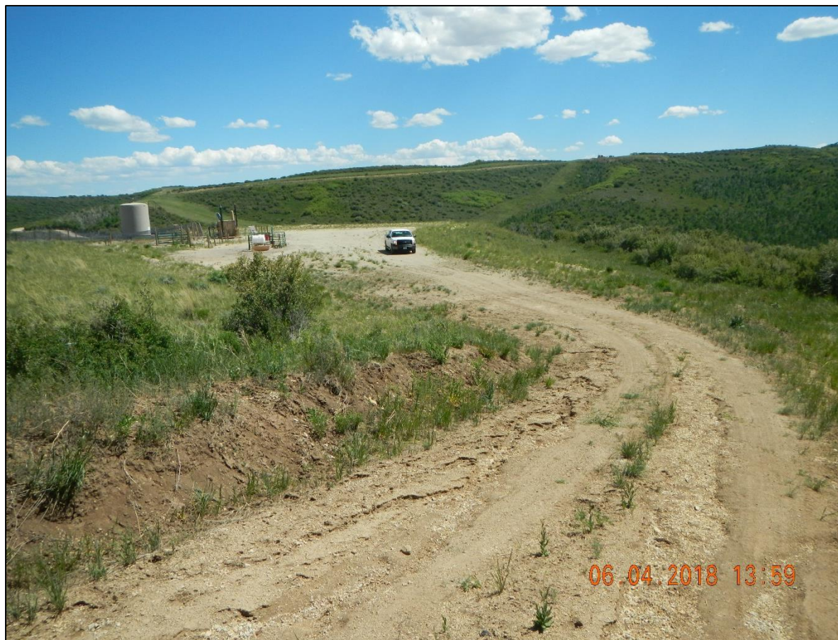
Washing and riling of rut on road. Sediment build up in ditch.
