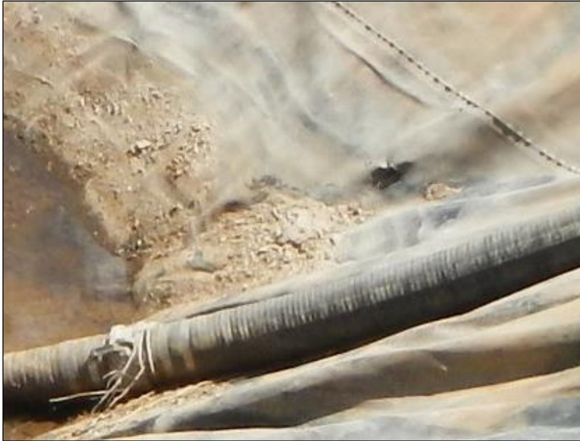
Tear in liner. (Close Up)
