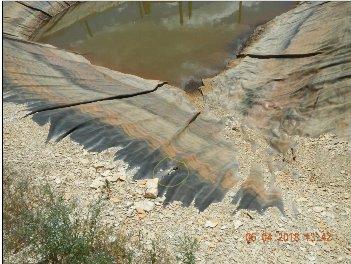
Tear in liner. (UP top in corner)
