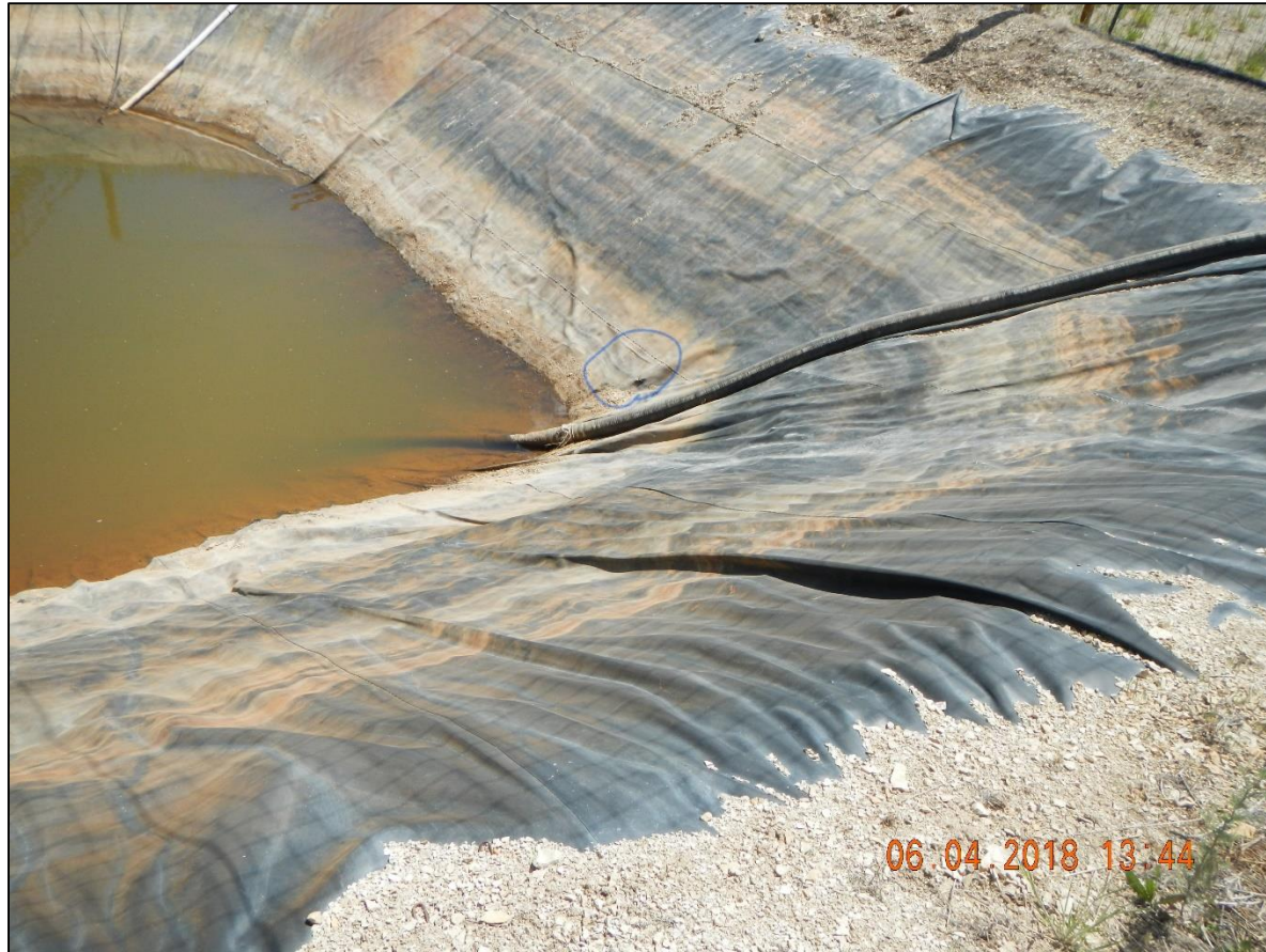
Tear in liner. (Just above fluid level by suction hose)
