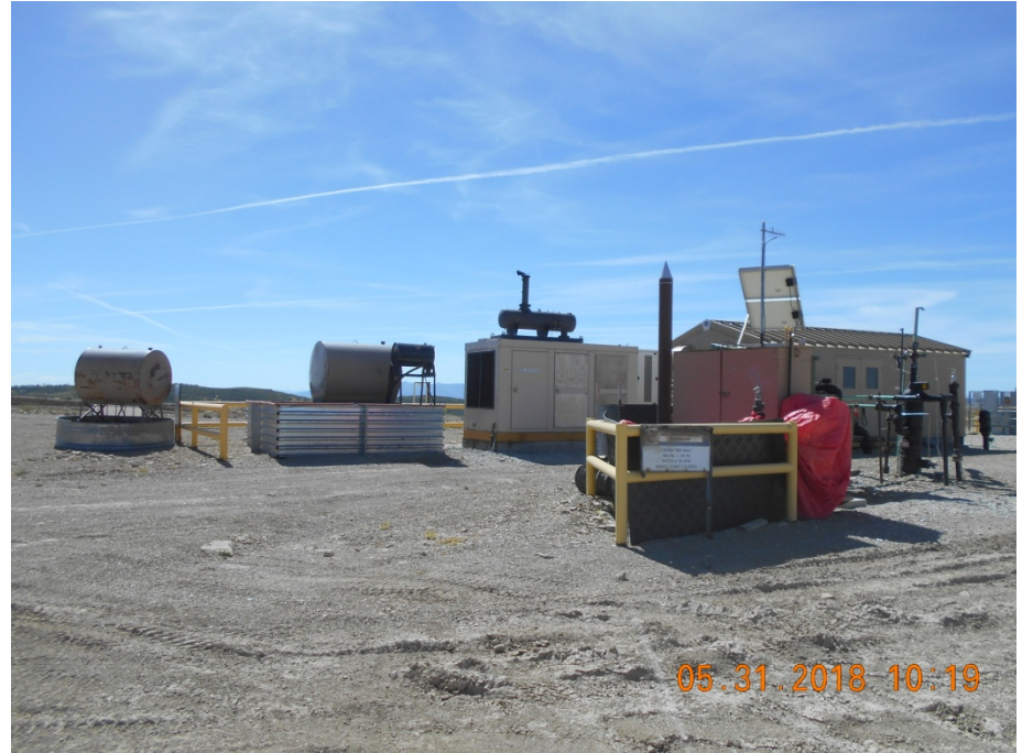
Pump housing, Meter shed, Separator and Generator
