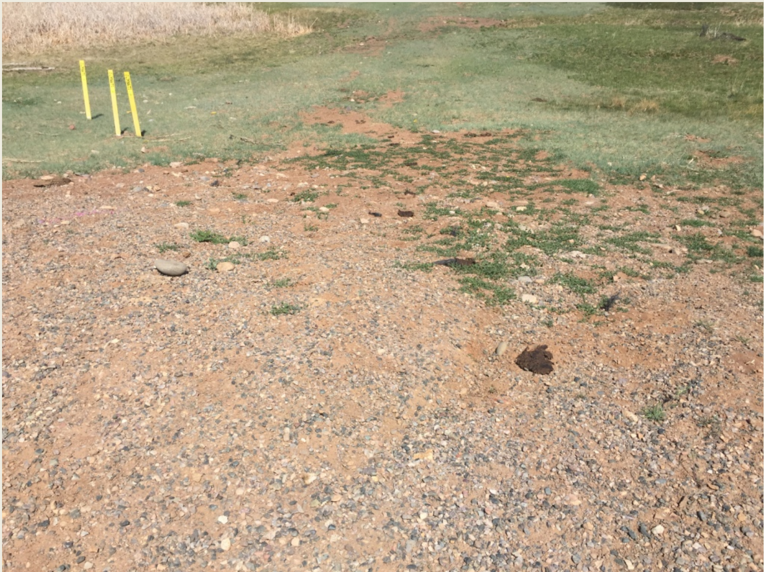
Photo 5. View of rilling along the pipeline alignment in the western project area.
