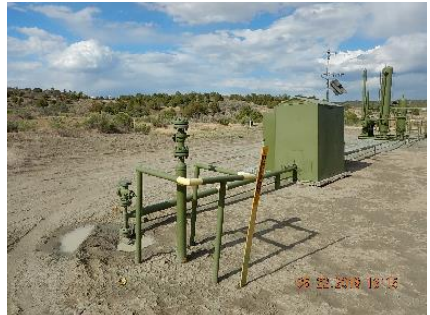
Photo 2: Unused steel riser with valve and cap..
