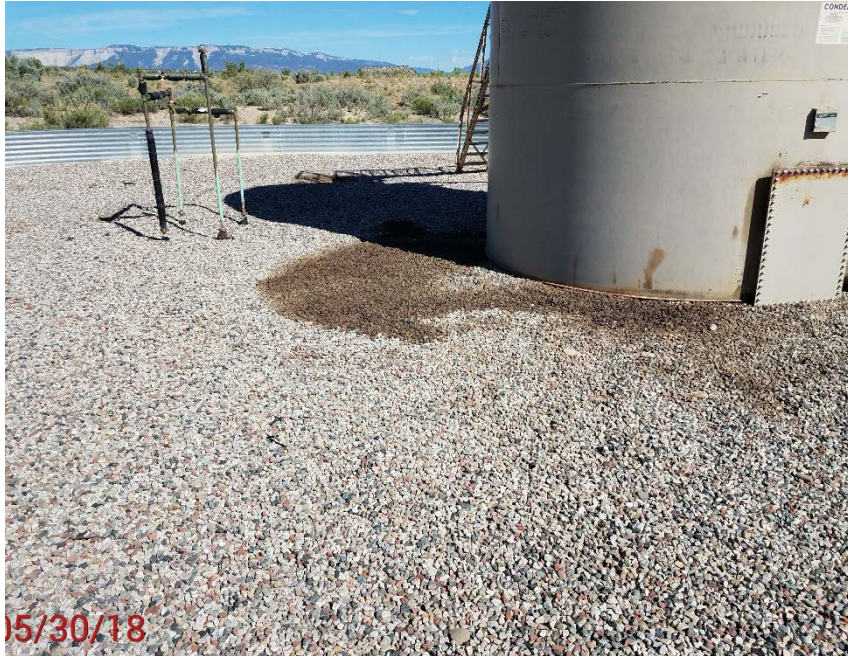
Location Photo #1, stained rock inside tank battery containment
