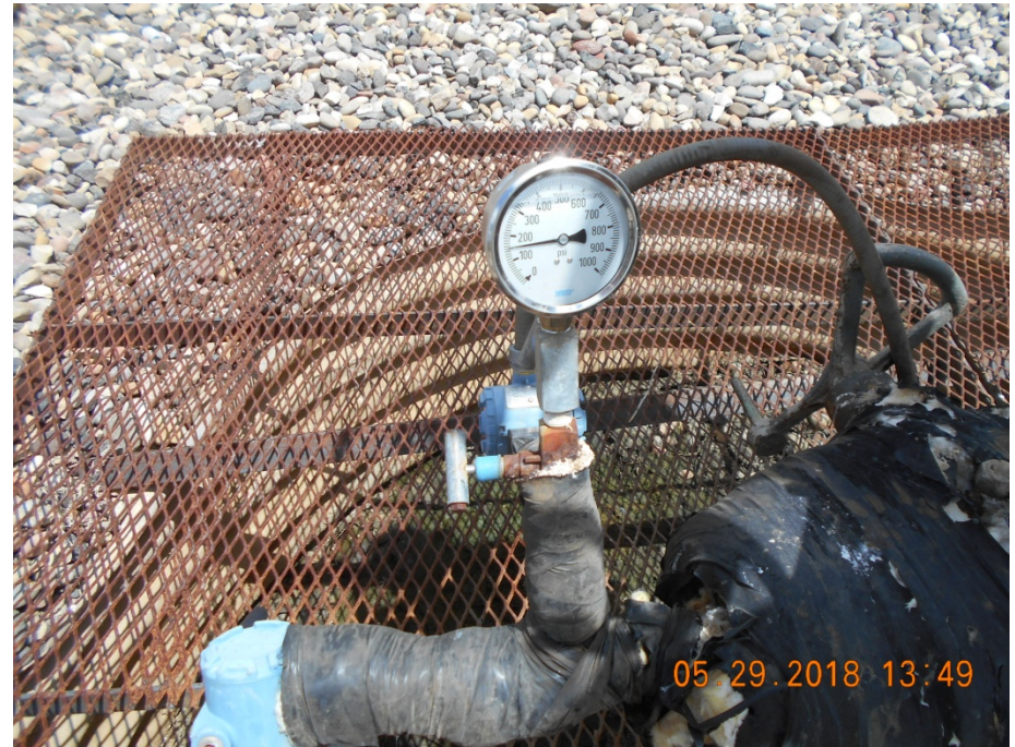
Injection wellhead casing gauge (150 psi)
