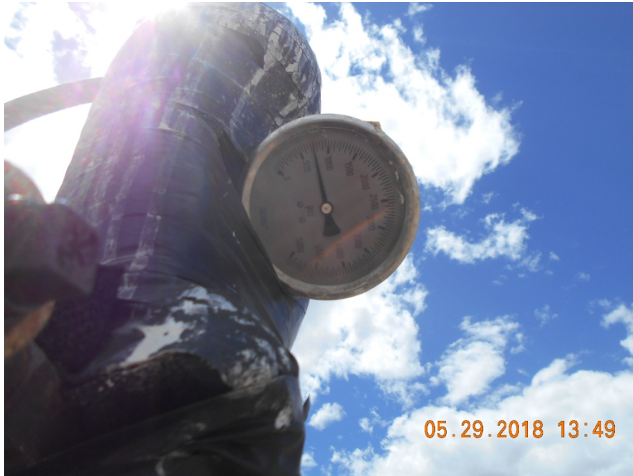
Injection wellhead tubing gauge (750 psi)
