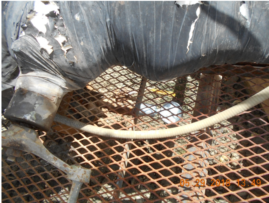
Injection wellhead bradenhead gauge (20 psi)
