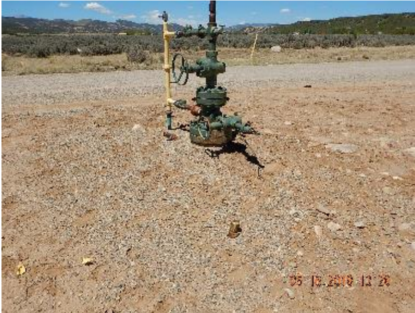
Photo 3: Unused 2" steel riser at wellhead.
