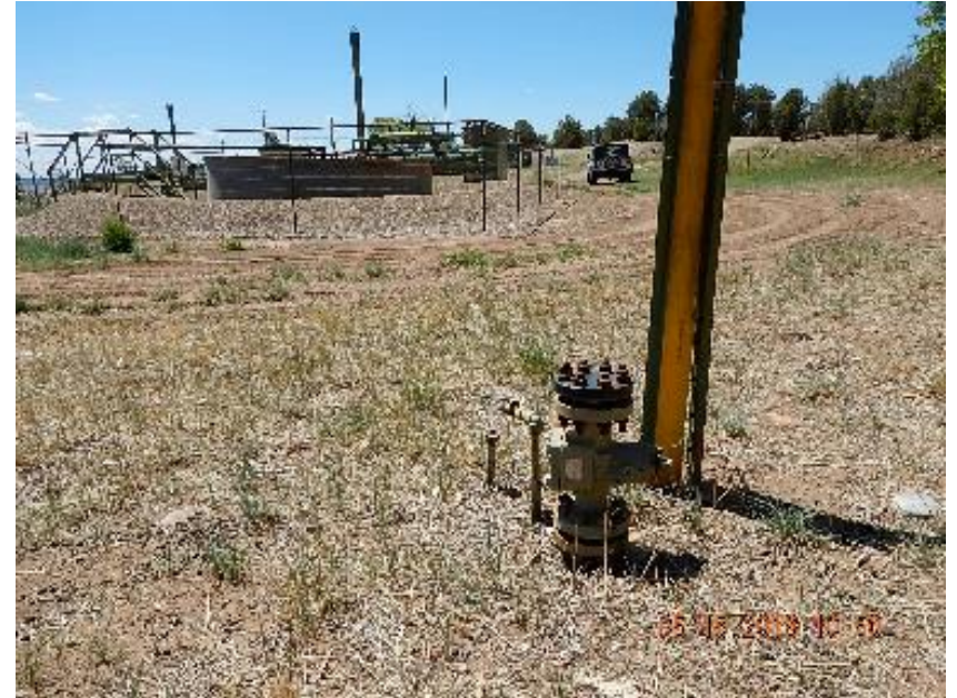
Photo 4: Risers in NW corner of location.
