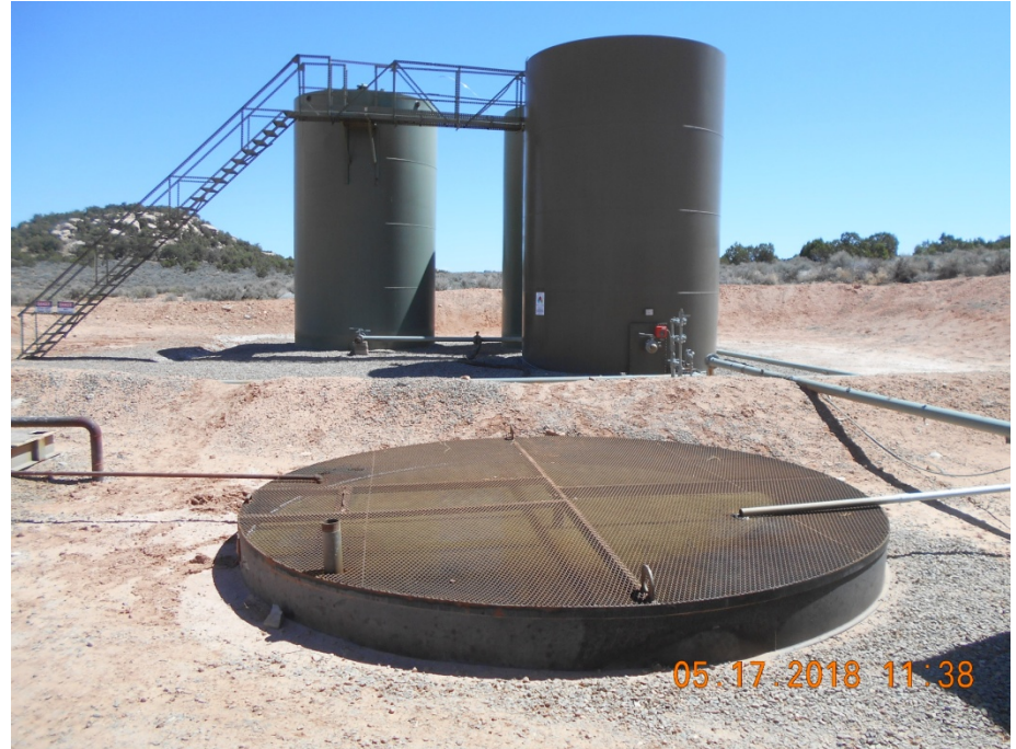
Tank battery and blowdown tank
