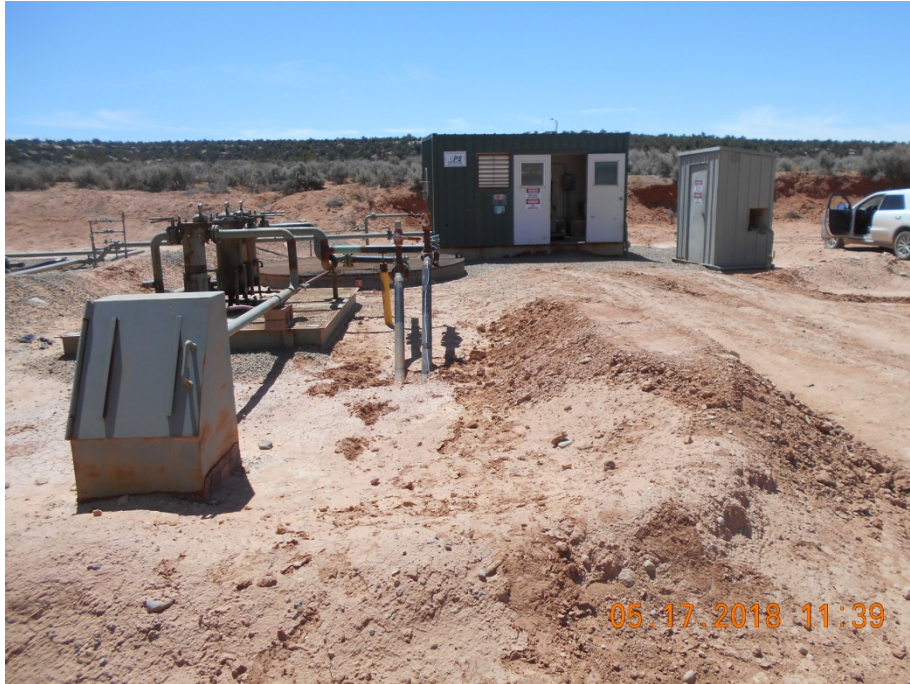
Pump housing, meter shed, filter pods and offload station
