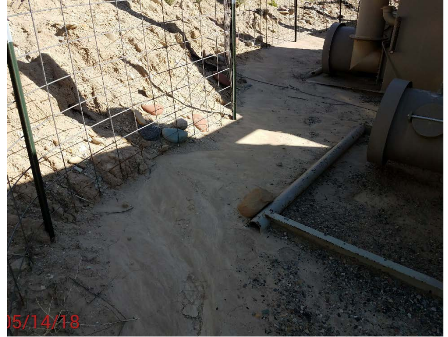
Location Photo #2, Storm water issue behind Separators
