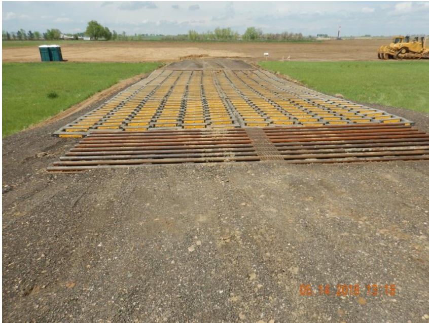
Photo 1. Photo taken from the entrance of location, facing North. Operator has installed tracking device BMPs. Based off the location file, Operator is not using the proposed access road. This access road is east of the proposed access road.
