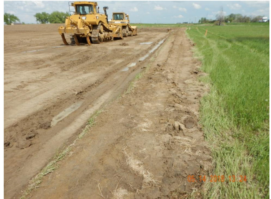
Photo 2. Photo taken from the entrance of location, facing East. Ditch and berm BMP has been installed around the entire perimeter of the location. Portions of the berm BMP are unconsolidated. An unconsolidated berm is not a proper functioning BMP.
