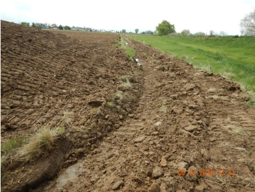
Photo 5. Photo taken from the northeast perimeter of the location, facing West. Photo illustrates a portion of the unconsolidated berm BMP and ditch BMP that need maintenance.
